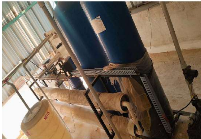
1000LPH RO Plant
