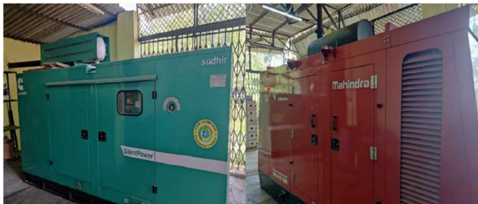
DG Generator Sets
