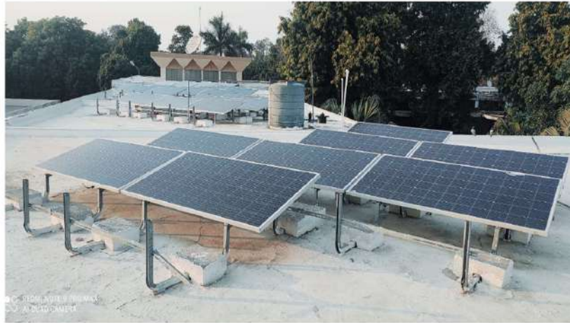
100 KW Solar Panels
