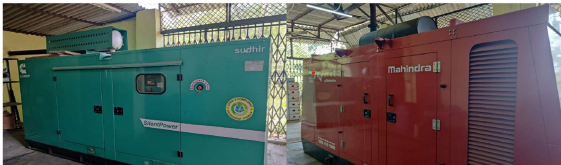
DG Generator Sets
