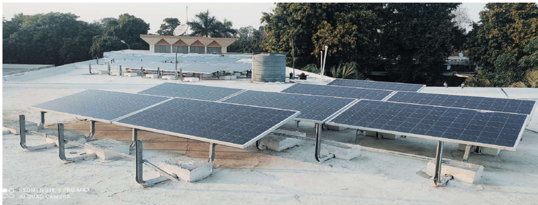
100 KW Solar Panels
