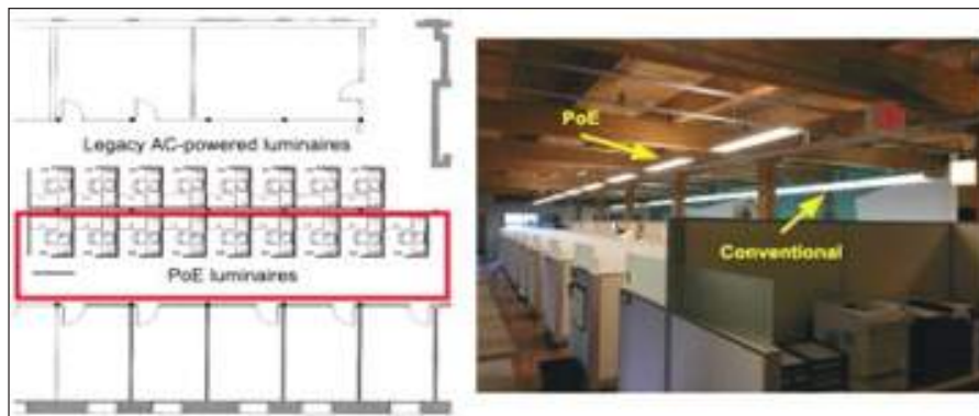
Fig. 3: Shows the Cubicles Layout with the Power Over Ethernet Luminaires and the AC Powered luminaire lighting Systems Along with a Photo of the Space
