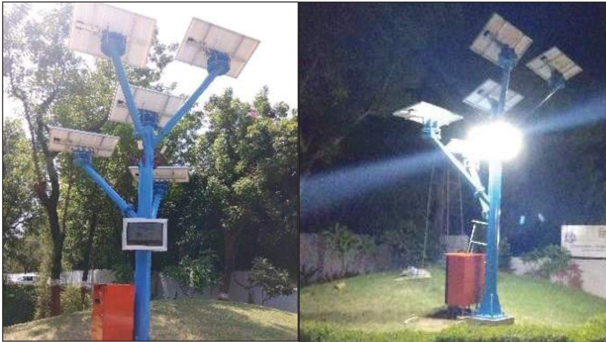
Fig. 8: Solar Tree Installed in the Park with a Street Light
